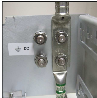
Fig. 11 – Termination of Grounding Cables
